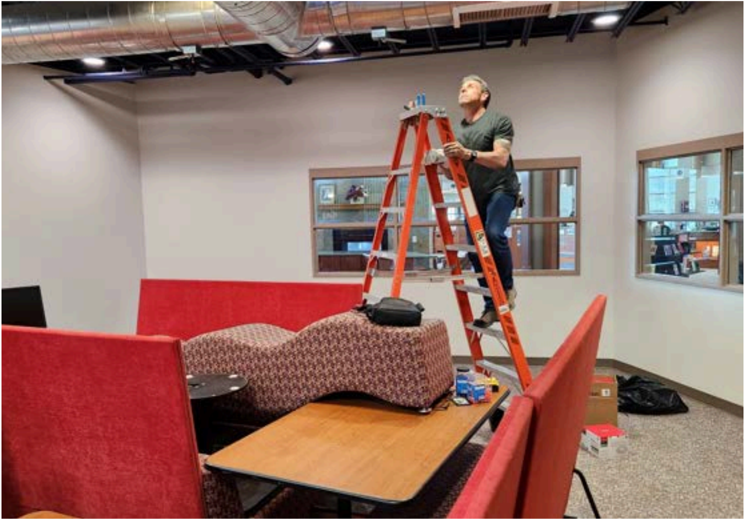
Andy Kareck from Facilities replaces some of our Teen Zone lighting with new LED fixtures.
